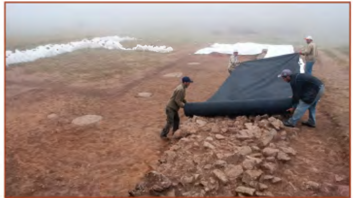
Figure 15. : Covering the walls with geotextile at the end of the excavation season.
