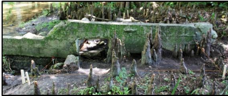
Figure 27. Profile view of trench01 showing new construction on top of older construction. Headrace is visible in center of picture.
