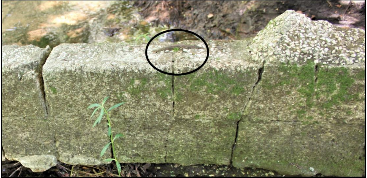
Figure 24. Visible metal reinforcement in concrete block on feature PMF07.
