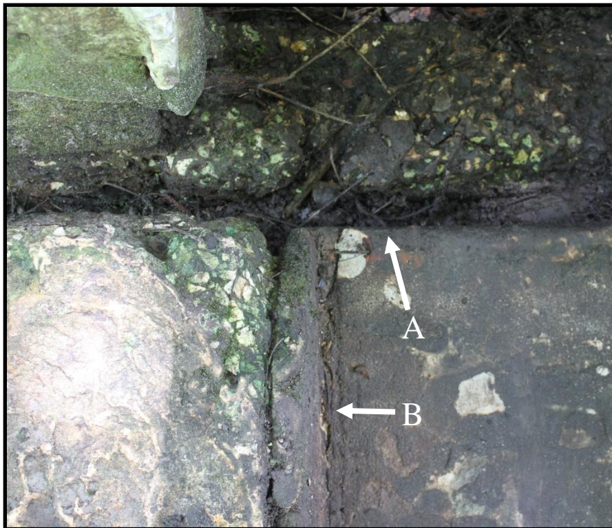
Figure 35. Headrace at opening to sluice. A, shows the area where the headrace and wall would have touched but not connected structurally. B, shows the support structure put in place to the north of the headrace.
