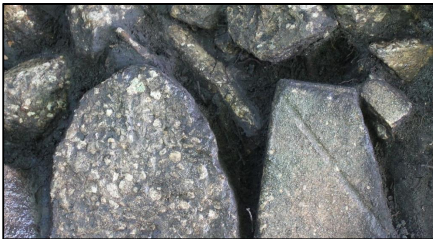
Figure 48. Wall Debris showing white stone aggregate and mold markings.
