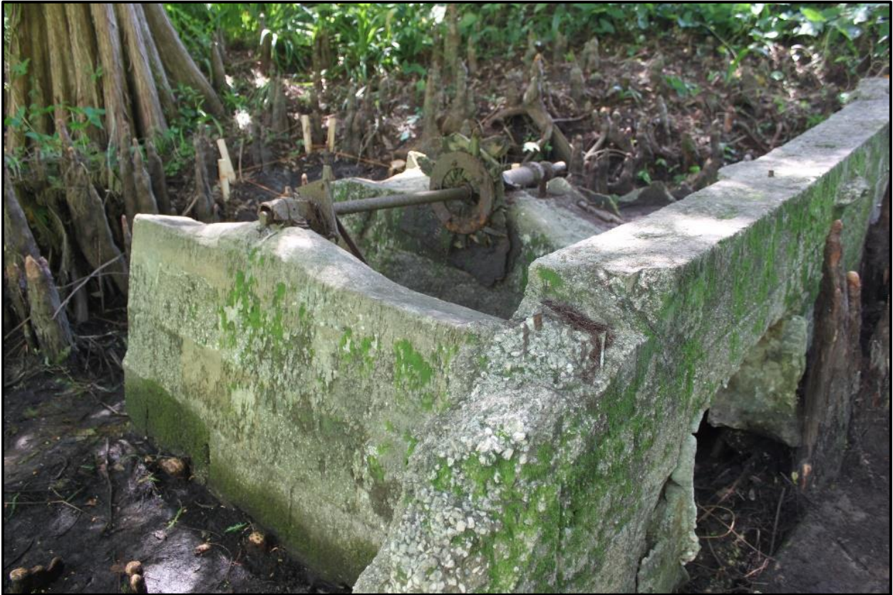
Figure 51. Headrace shown on the right connects to the sluice below the center of the wheel or in this case the observable axle.
