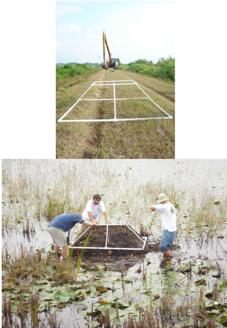
Figure 4. (Top) District personnel used heavy equipment to pile submerged marsh soil into artificial islands, which were shaped using the white frame (foreground). (Bottom) Dr. Quintana-Ascencio and two members of the Biology Graduate Student Association shaping willow islands.
