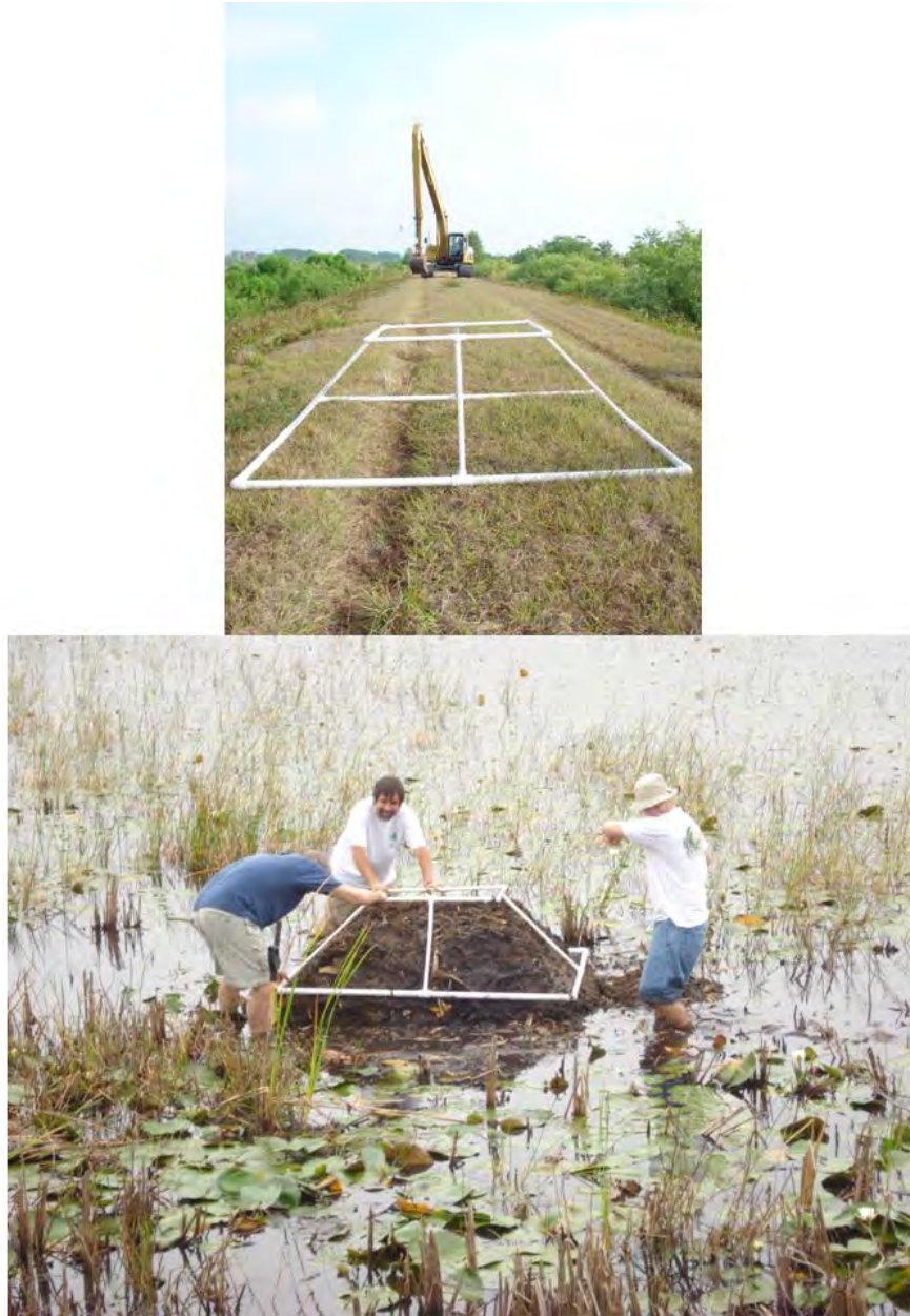
Figure 21. (Top) District personnel used heavy equipment to pile submerged marsh soil into artificial islands, which were shaped using the white frame (foreground). (Bottom) Dr. Quintana-Ascencio and two members of the Biology Graduate Student Association shaping willow islands.
